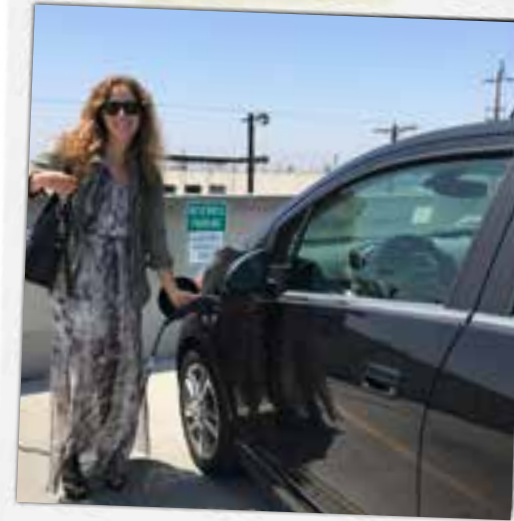
EV charging station at Los Angeles headquarters
